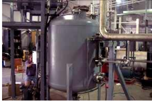
Tank and blower
