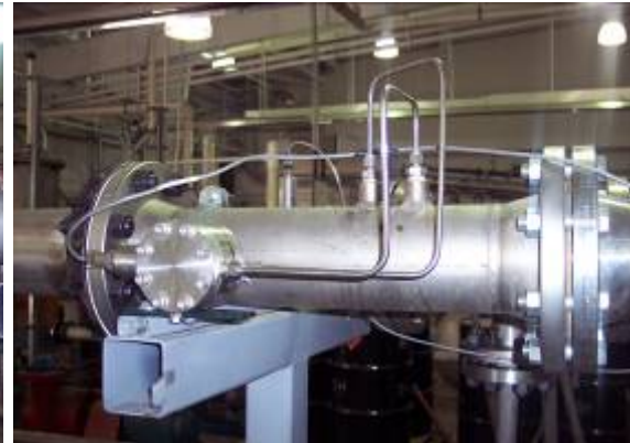
Gas flow meter
